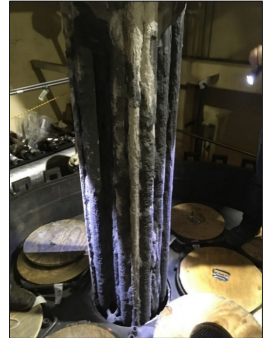
Process Gas Filter - filter bundle - caked
