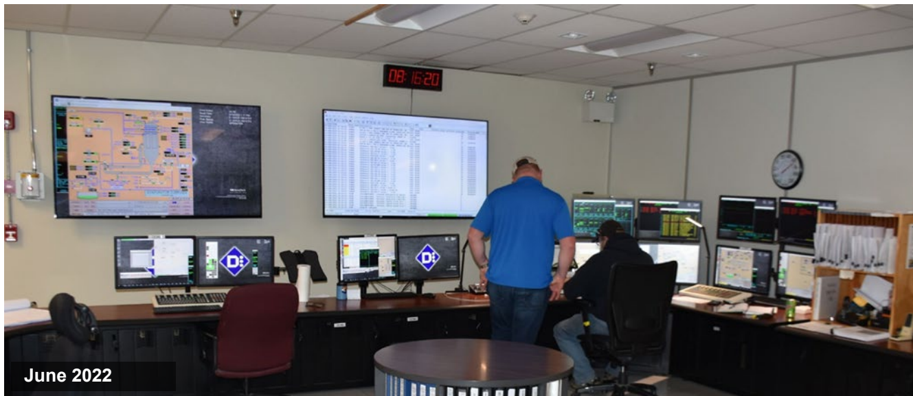
242-A Evaporator monitoring and control system
