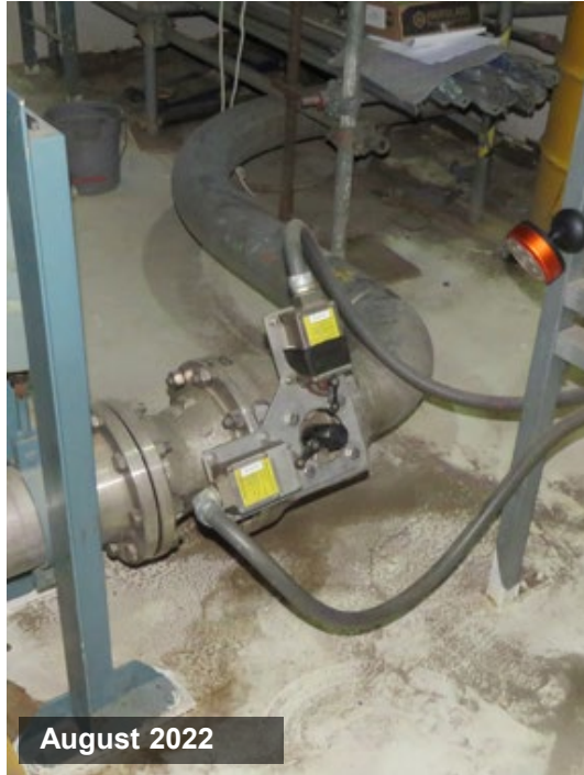
Dump valve in the evaporator room
