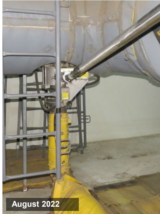
Dump valve in the evaporator room
