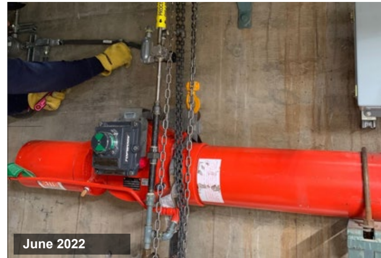
Valve actuator in the condenser room
