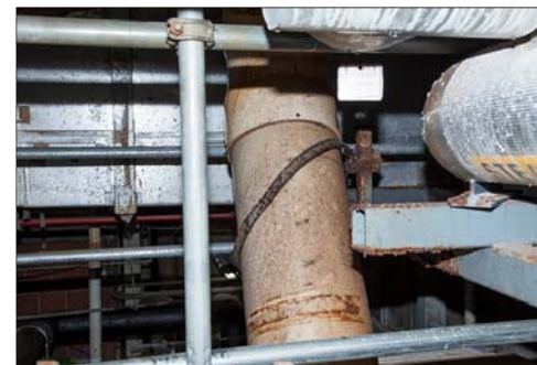
Y-12 Kathabar System Failure
