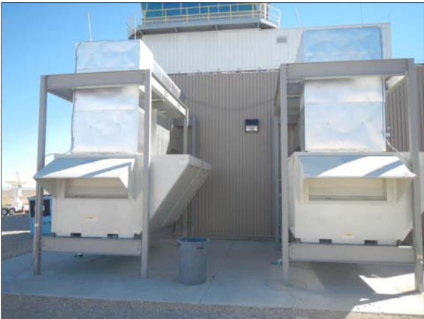
SNL Tonopah Main Distribution Hub
