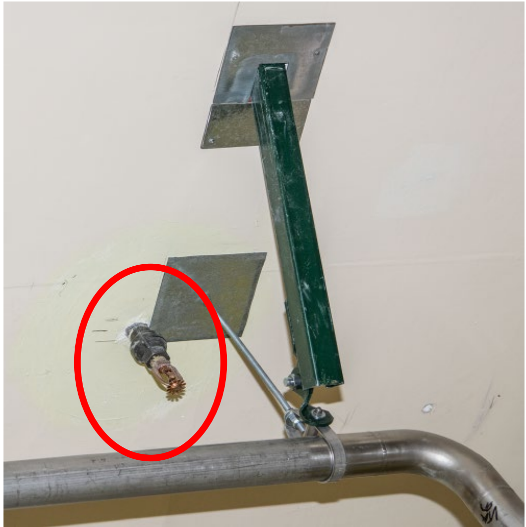
Sprinkler head on the ceiling of PF-4.
