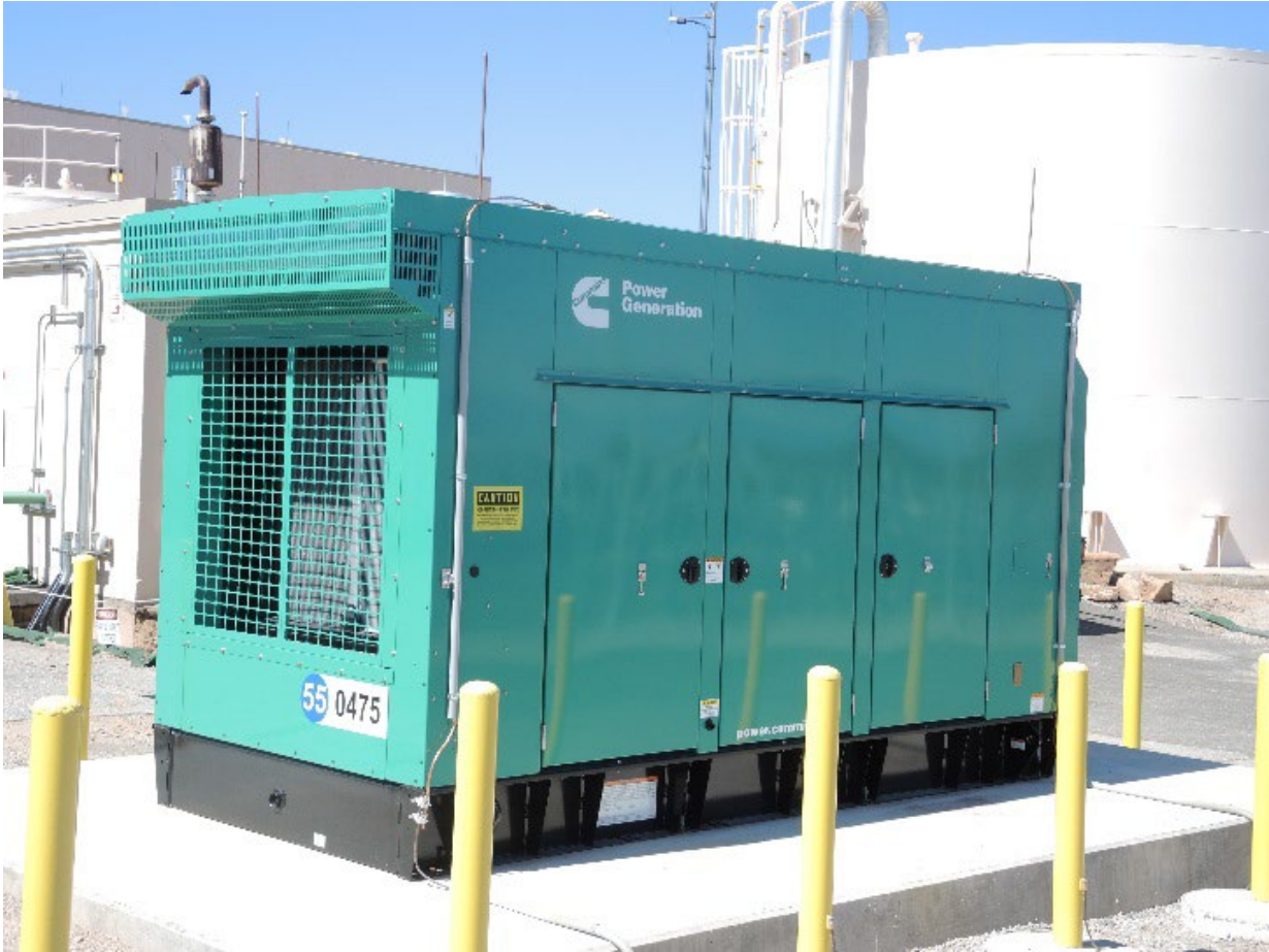
Generator for electrically-driven firewater pump.
