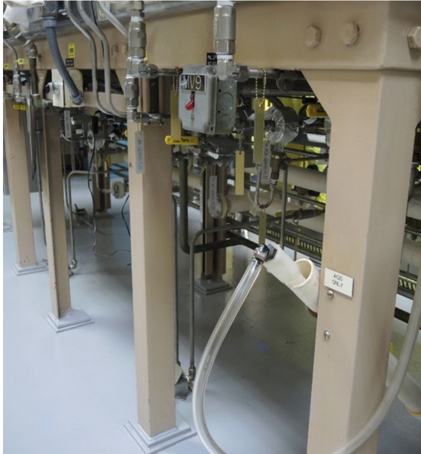
Seismically-deficient glovebox stand used for plutonium solutions.
