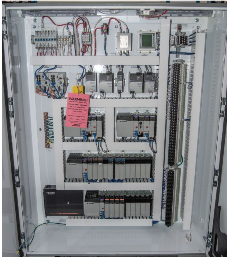
Components of the Facility Control System.
