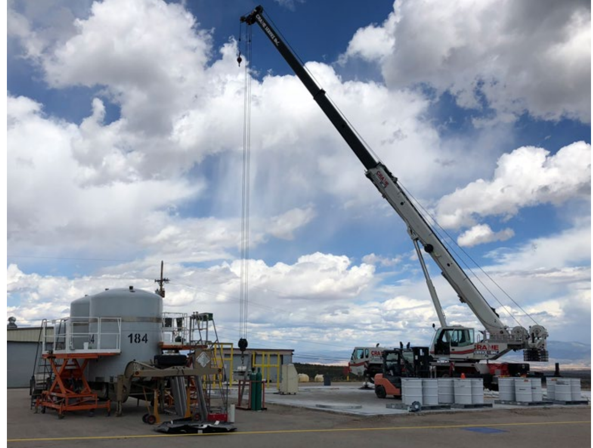
Mobile Loading Unit at Area G.
