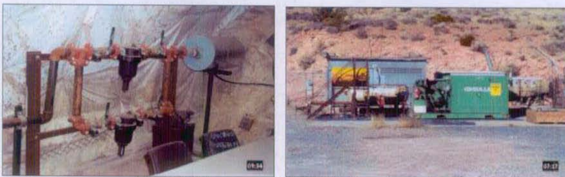
Figure 5-6. Compressed air for U12g Tunnel operations.
