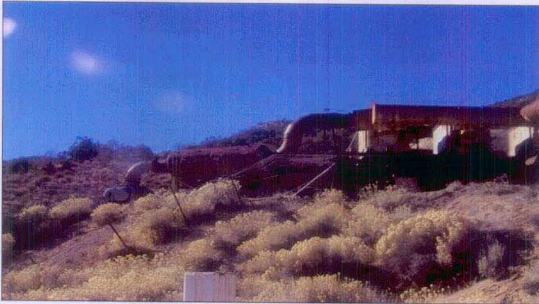
Figure 4-1. Dual 300-hp Sutorbilt Ventilation Fans.
