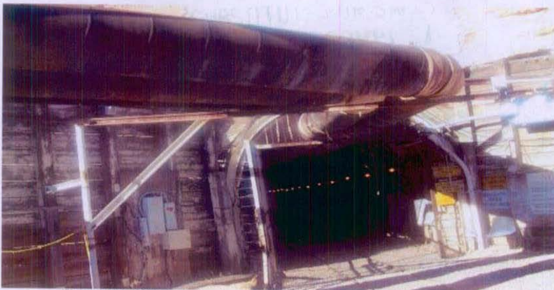
Figure 4-2. 30-inch duct network originating from the tunnel portal entrance.
