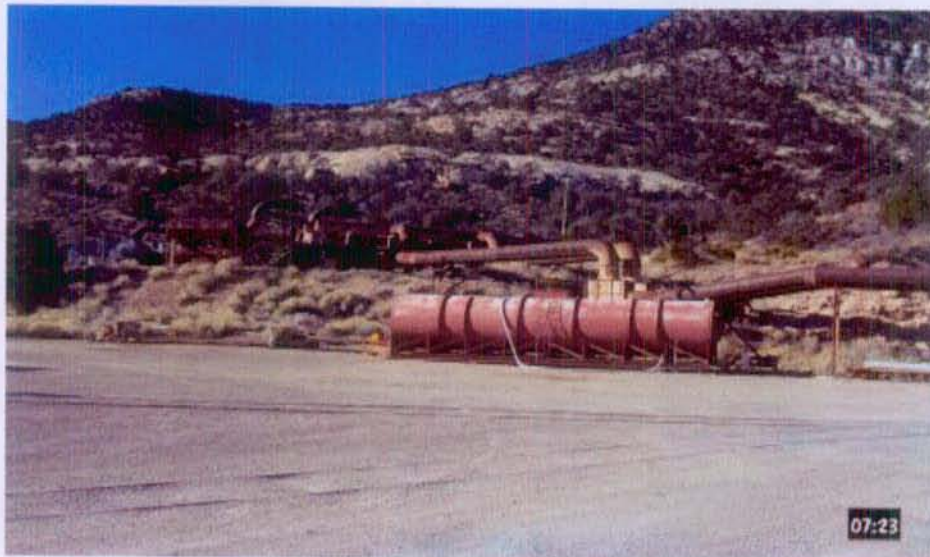
Figure 5-7. U12g Tunnel 16,000-gallon water tank.
