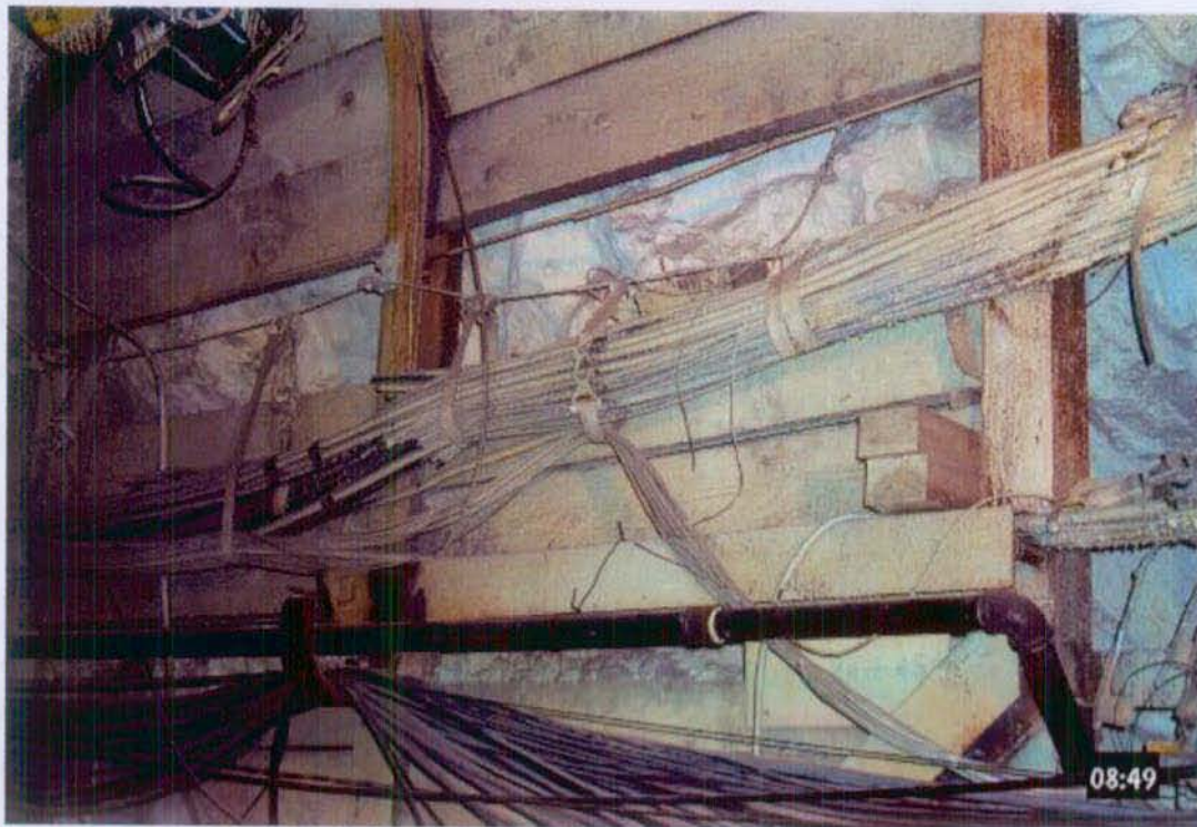
Figure 4-7. Abandoned electrical wiring scheduled for removal.
