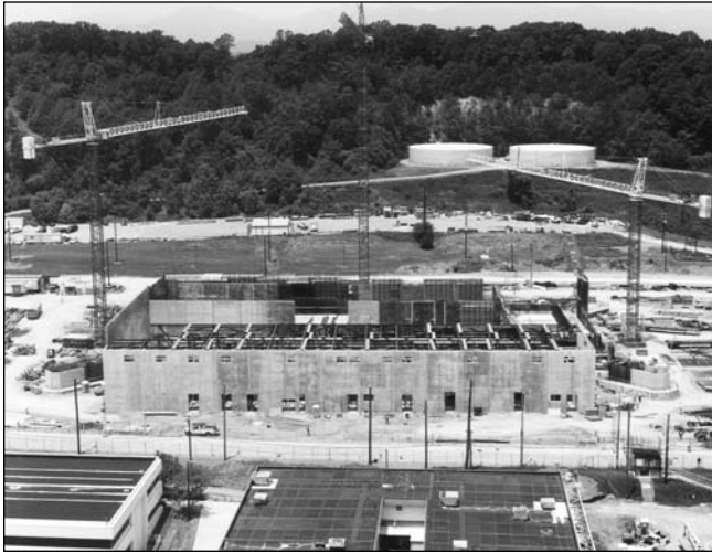
View of the Highly Enriched Uranium Materials Facility under construction at Y-12
