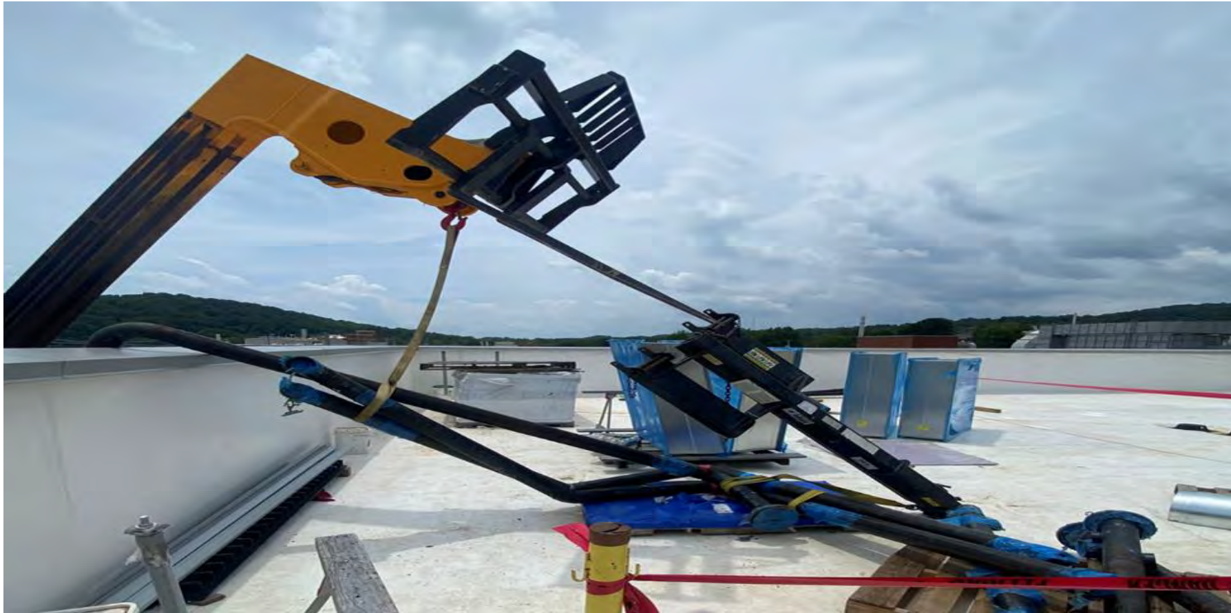
Telehandler, Jib, and Load on Roof Post-Incident
