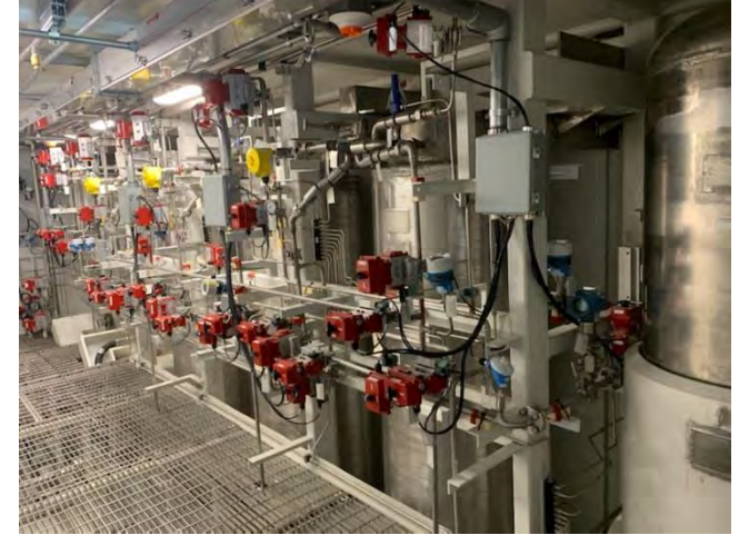
Tank Side Cesium Removal System Process Enclosure
