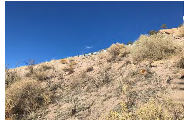
Cliff Alongside Transportation Route in Los Alamos
