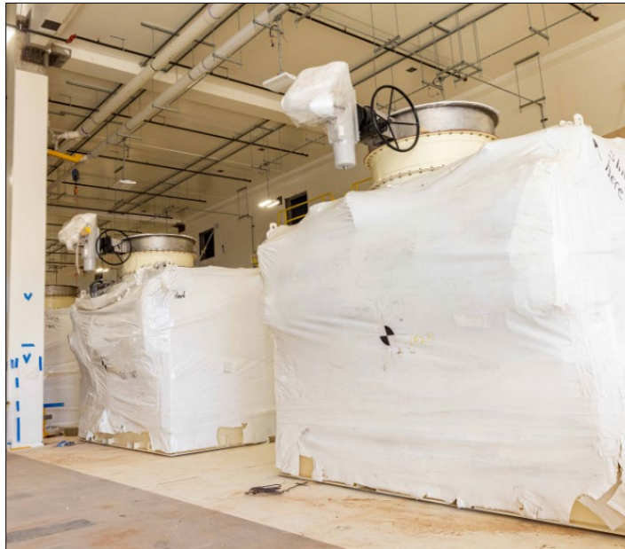
Figure 23. Filter Housing Assemblies Inside the New Filter Building
