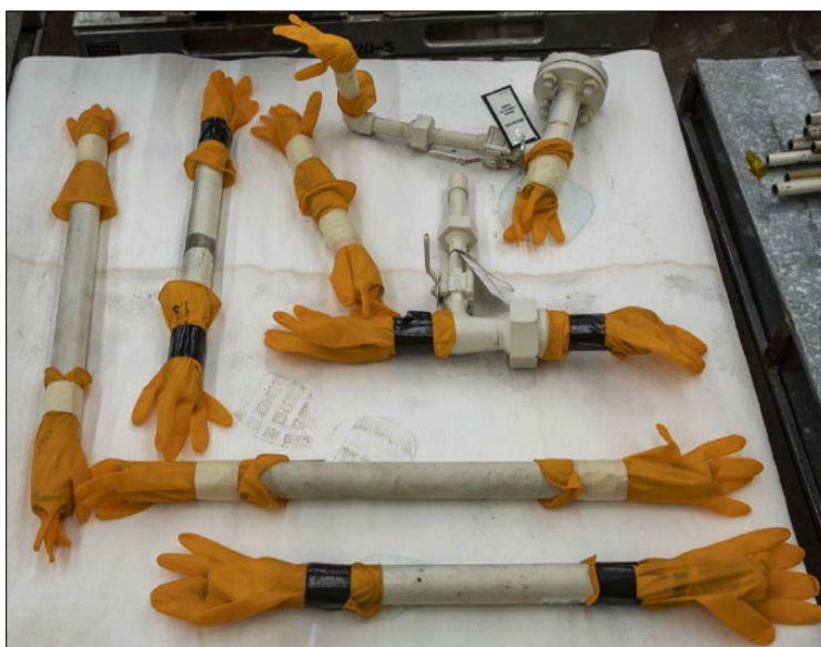
Figure 6. Machine Coolant Piping Capped with Rubber Gloves
