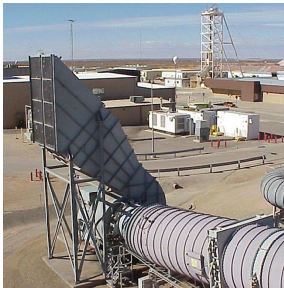
700-C Exhaust Fan under Preparation for Restart
