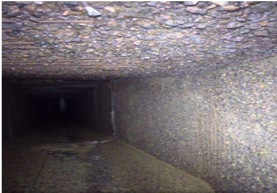
HCAEX Tunnel Concrete Surface Degradation as of 2018
