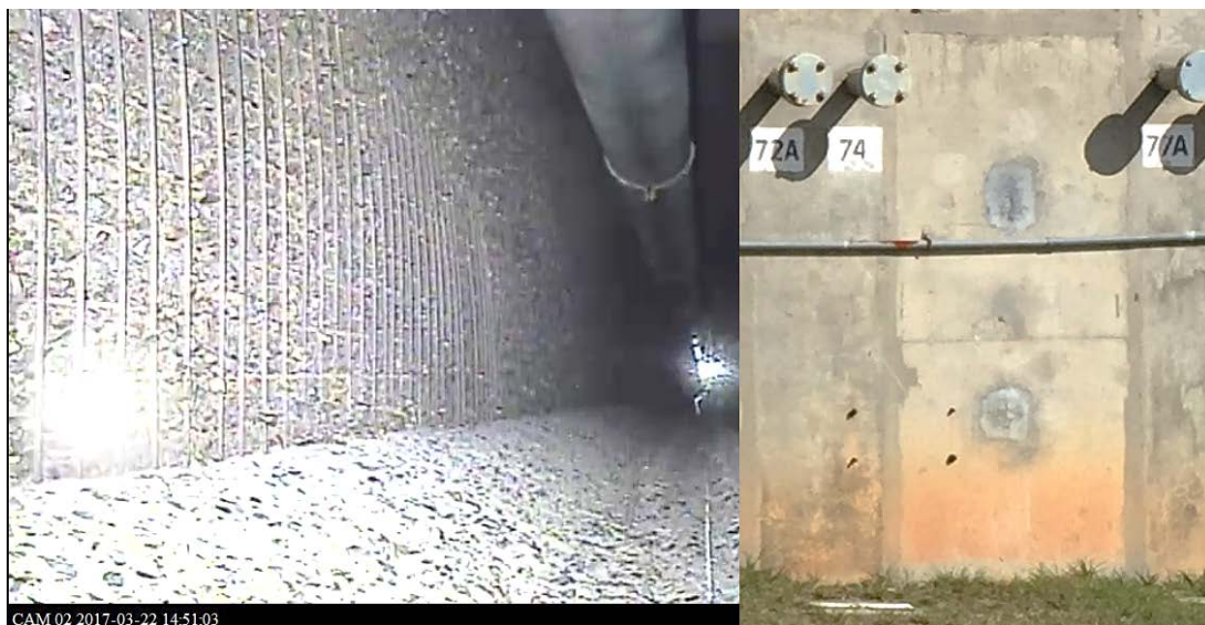
Figure A-2. Comparison of a still from the 2017 crawler inspection video of inside HCAEX Tunnel (left), and a set of two coring locations on the exterior wall of the H-Canyon Facility (right).
