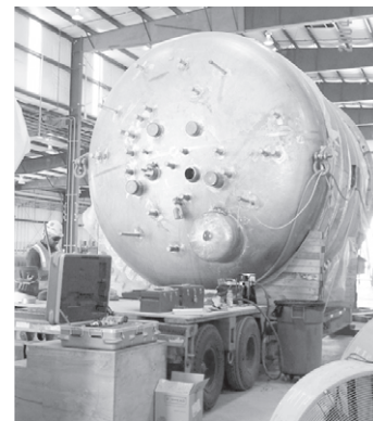
The pipefitter is working on the nozzle for the High-Level Waste Facility located at the Office of River Protection.
