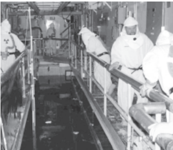
Team members of the K Basins Decontamination and Decommissioning project begin pouring grout to permanently fill and secure the discharge chute.
