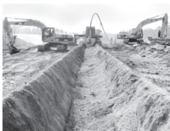
Hydrologic isolation activities for Solid Waste Storage. This includes employing a state-of-the-art trenching technology that ensures that the project meets the regulatory requirements for reducing groundwater infiltration into the Waste Burial Grounds at Y-12.
