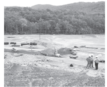
Solid Waste Storage Areas undergoing remediation on the Oak Ridge Reservation in Oak Ridge, Tennessee.
