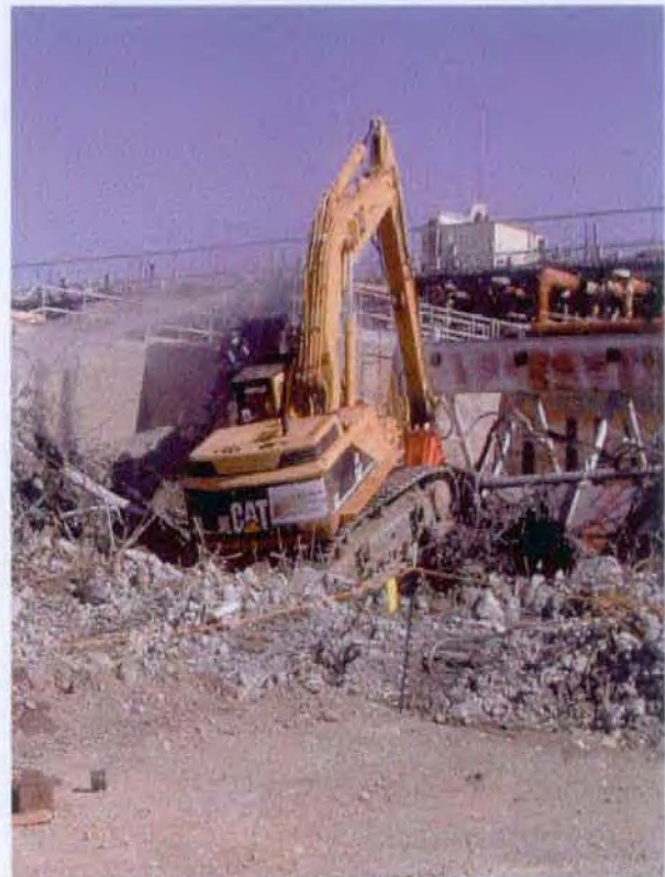
A Support Building for Hanford's N Reactor Is Being Demolished. It Is One of Hundreds of Surplus Facilities That Will Be Demolished as Part of the River Corridor Closure Project
