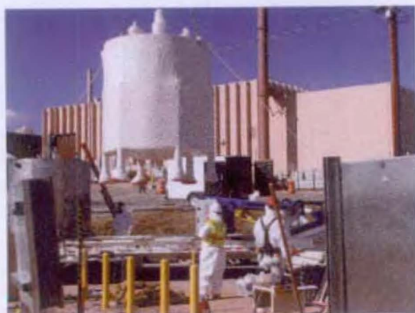
Workers Remove the 20+ Year-Old Caustic Tank at TA-50 Rad Liquid Waste Treatment Facility
