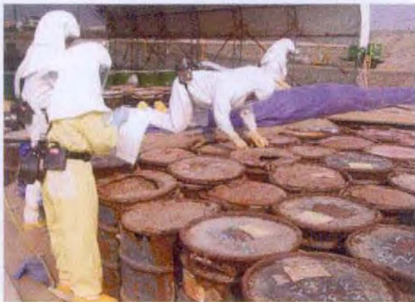
Retrieved Buried Waste—the First 21,300 of 75,000 Drums of Radioactive Material—Five Months Ahead of the Regulatory Milestone
