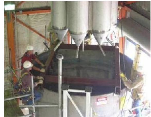
Typical arrangement of multiple pulse jet mixers in a WTP pretreatment vessel
